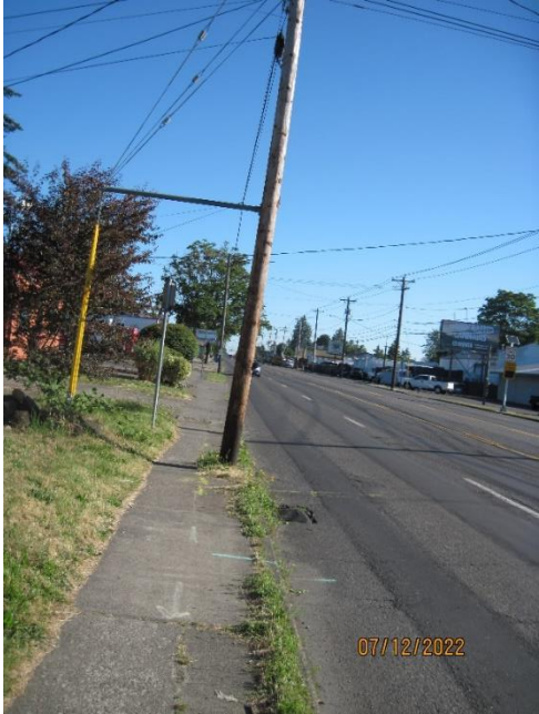
Curb-tight, narrow, dangerous section of sidewalk on 82 nd Ave. Photo by Bruce Nelson.
